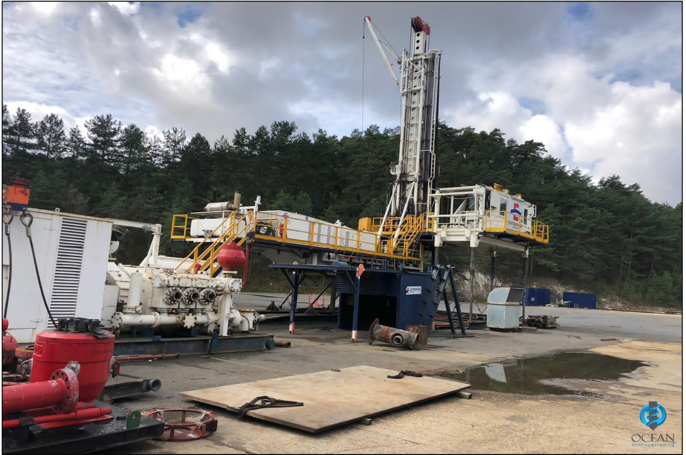
DRILMEC Drilling Rig 270 ton pull back With all equipment ready for job
