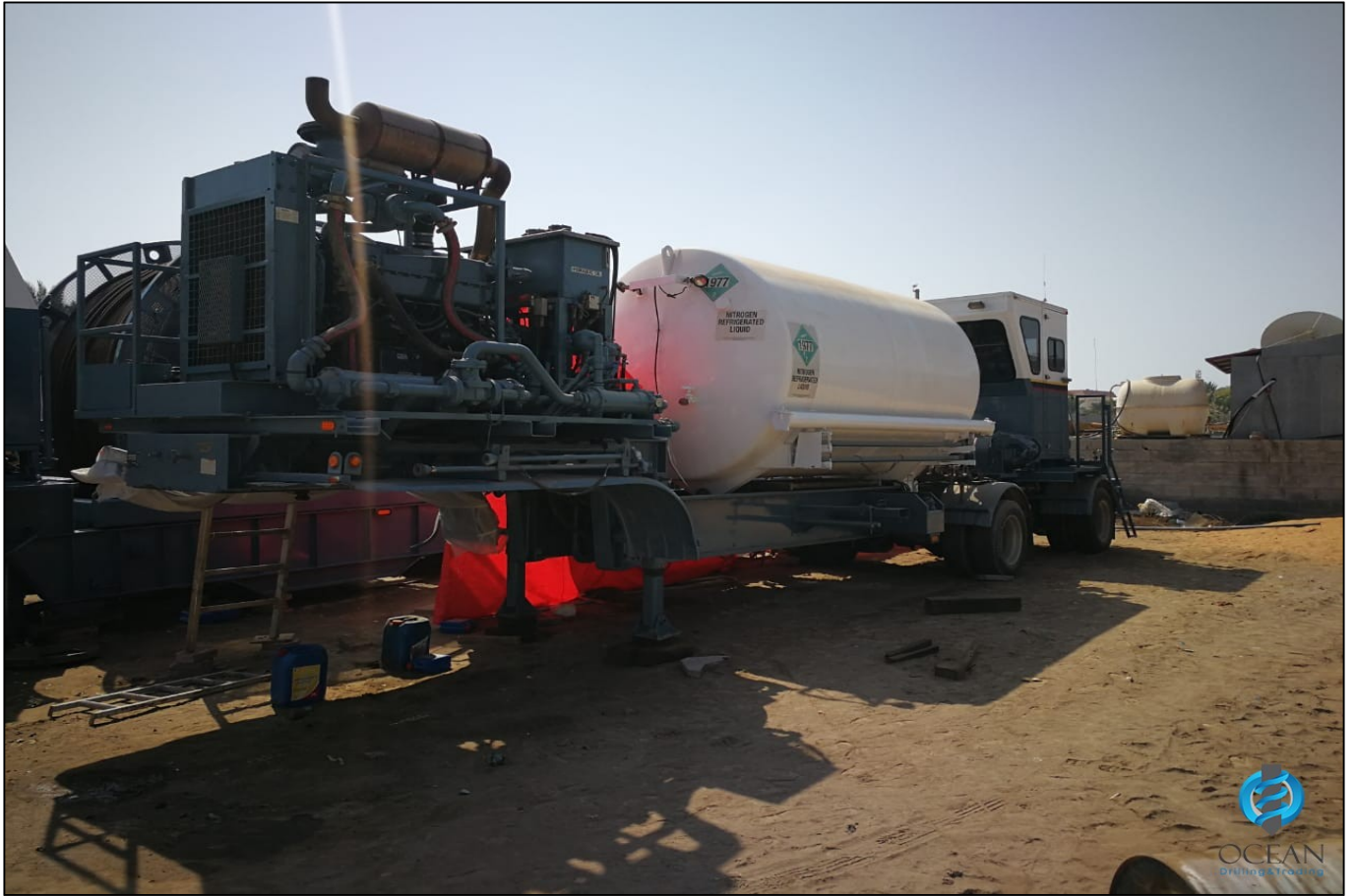
Nitrogen pump unit
